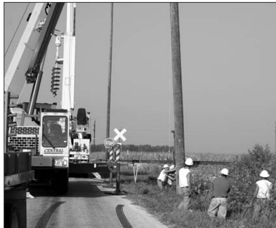
REMC crews use a crane to help set an extra tall pole for a railroad crossing the plant will utilize.
